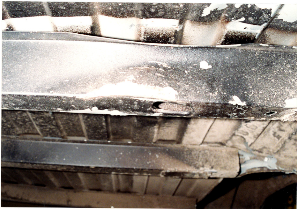
18. Close-up view of the cargo bed transverse strut showing the indentation from contact by the failed CNG tank
